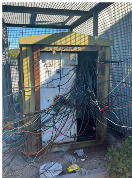
Figure 4: Informal electricity connections, Cape Town
